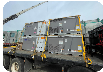
New high efficiency HVAC units
